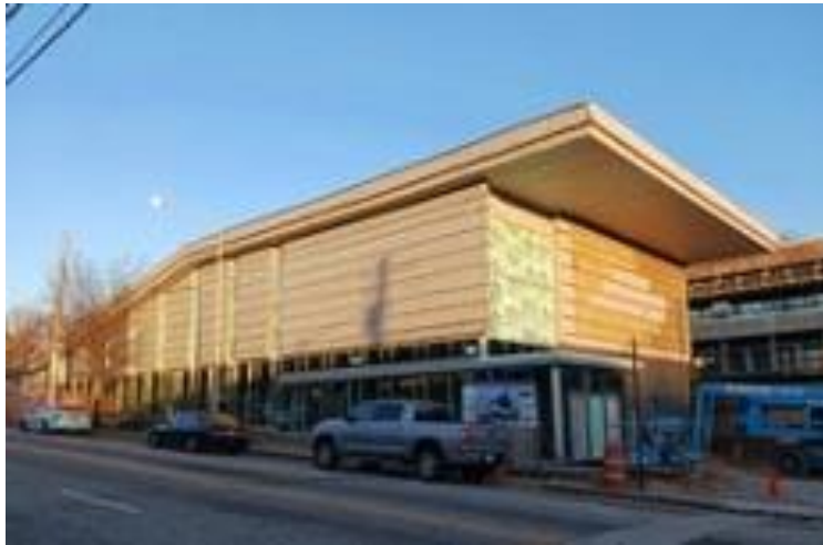
Atlanta's new Greyhound Bus facility being built with financial support from the state government.
